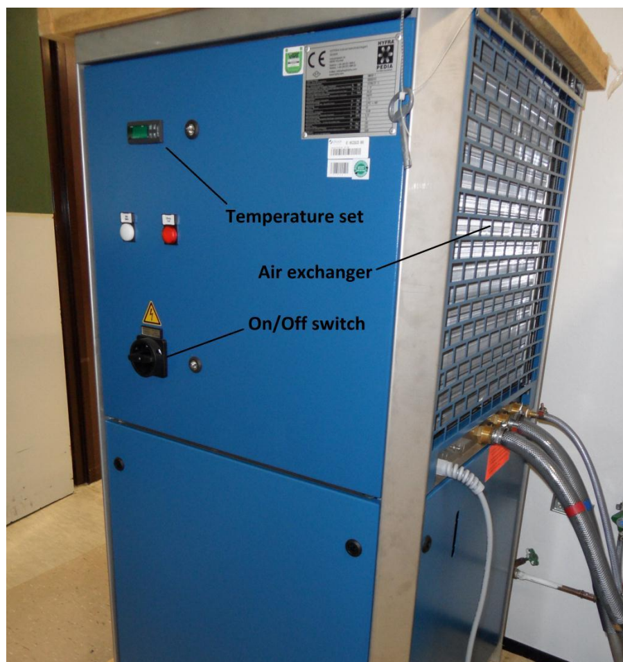
Figure 4.2.4: Overview of the cooling unit
