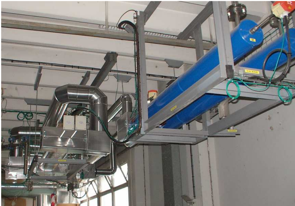
Electrical heaters of circuit 600 : Heater 600 et Heater 601
