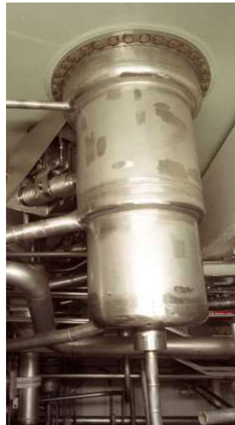
Figure 21 - Mixer settler in a nuclear installation [24]
