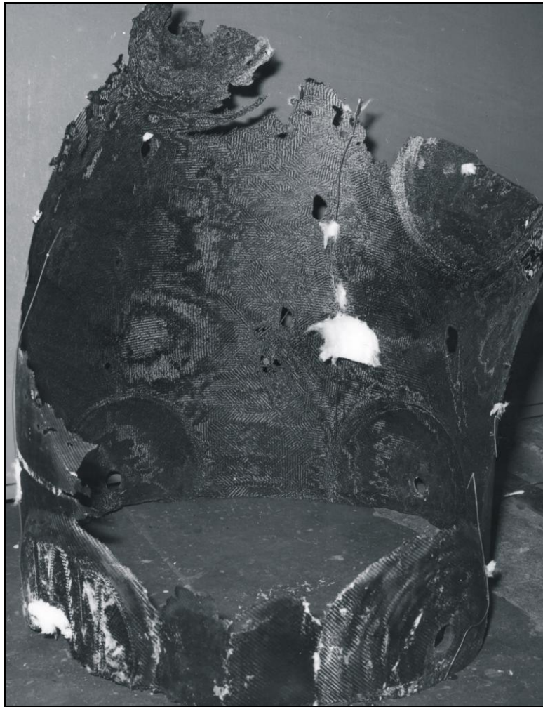
Figure 116: Destroyed ducting shroud
